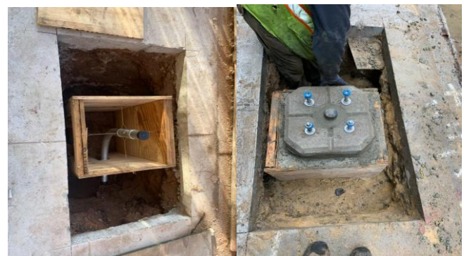
Lightpole foundations installations on E.25 th St. between Lexington Ave. to 3 rd Ave.
