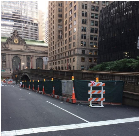
Green mesh netting covers the construction materials storage yard on Park Avenue at 40 th Street.
